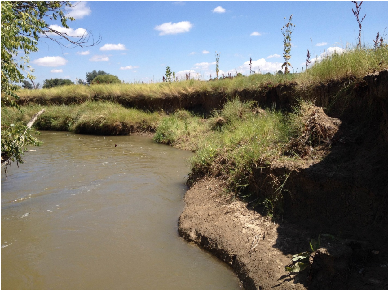
Photo 10, Reach 6A: Failed blocks of bank material temporarily protect the bank from further erosion. View looking downstream.
