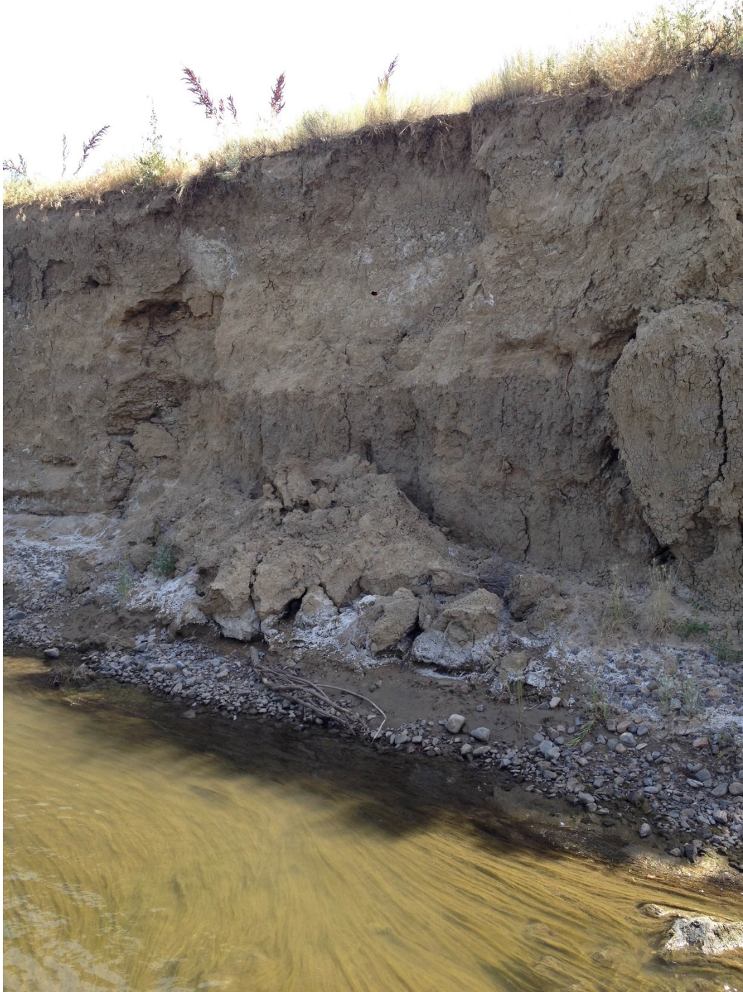
Photo 6, Reach 3C: A recent bank failure. Wetting-drying cycles appear to be weakening the bank material, making it more susceptible to fluvial erosion and mass failure. Flow direction is right to left.
